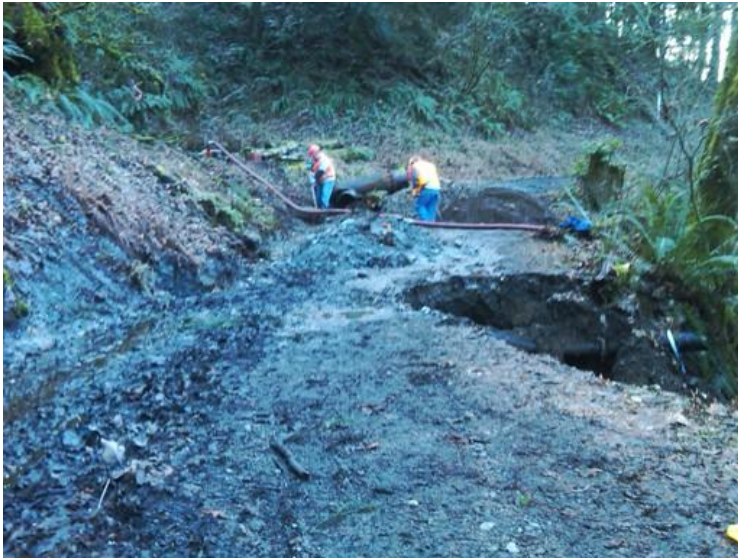
City crew working to remove the damaged and clogged drainage culvert to make emergency repair.
