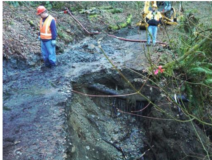
Area of trail washout beyond the culvert repairs.
